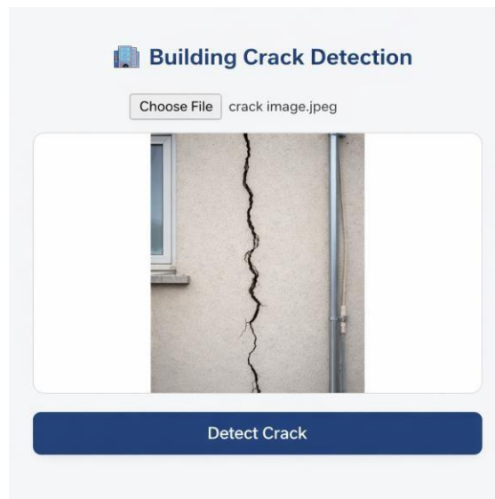
Fig. 2. Crack Detection Results Screenshot
